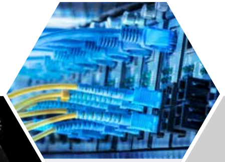
FIBER OPTIC CABLES
